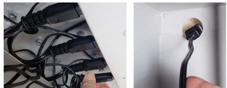
1. Securely connect the new Power Cord connectors to each of the six Chargers.
